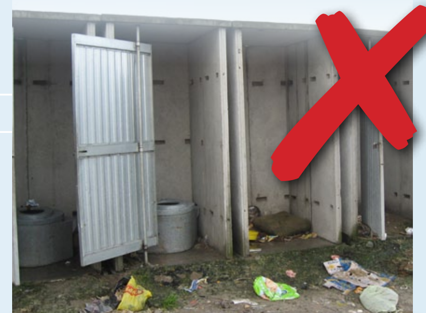
Do not block drains or vandalise toilets
